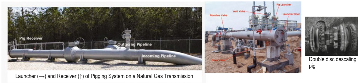
Figure 3.20 Pigging System. (Source: Metropolitan Engineering Consulting & Forensics brochure, 2008)
