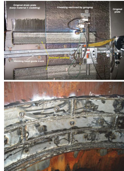
Figure 4.75 Weld overlay repair welding on Cr-Mo coke drum (Horizontal SAW Process) – source: API RP572 and others
