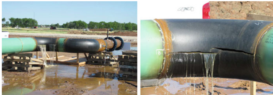
Figure 5.35 Failure during hydrostatic leak test of pipe spool. (Source: Hanging H Co.)
