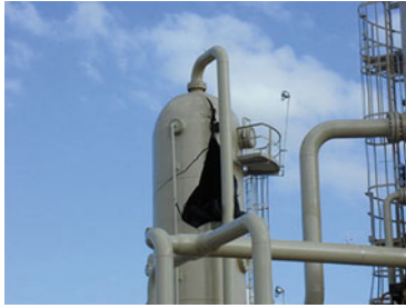
Figure 1.48 Failure due to pressuring under limitation of low temperature during startup. (Source: CLG report 2011)
