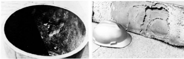
Figure 2.178 Naphthenic acid corrosion accelerated on high-temperature sulfidation corrosion. (Source NiDI Publ.9021)
