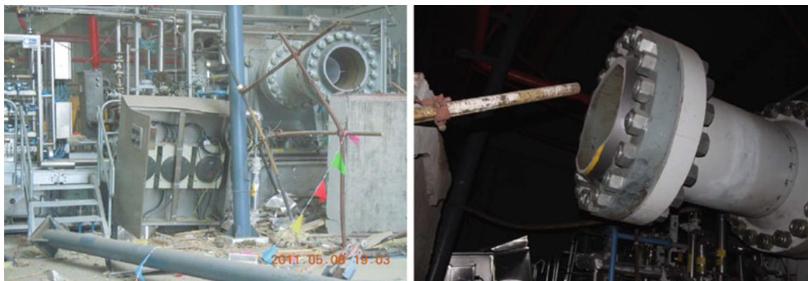
Figure 5.38 Failure during nitrogen pressure test in LNG tank terminal
