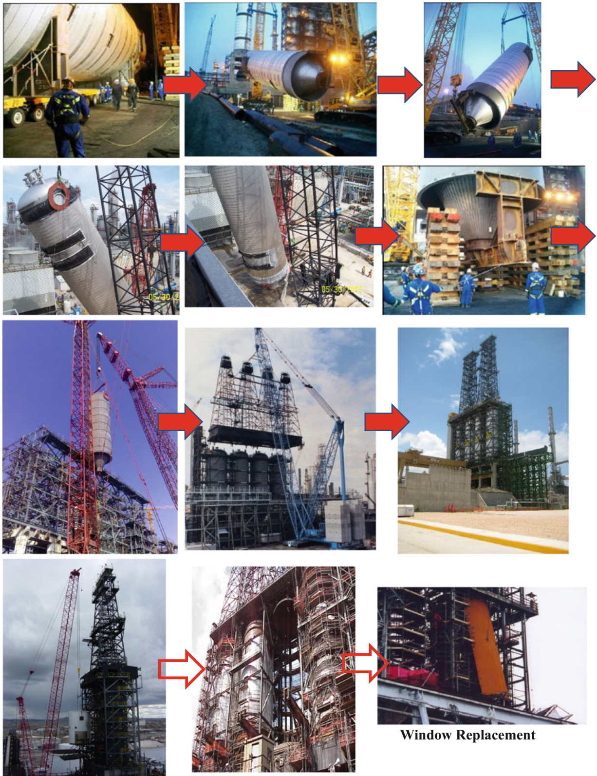
Figure 3.7 Erection sequence and replacement of coke drums in delayed coker unit of refinery plants
