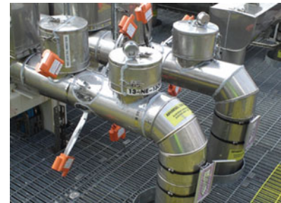
Figure 5.26 UT sensors installed in the piping. (Source: Inspectioneering Journal, p1–6, Jan./Feb. 2016)
