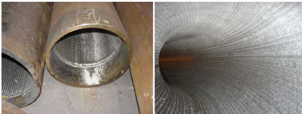
Figure 4.72 Weld overlaid surfaces in pipe and elbow
